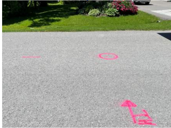
June 2022 - Completed test pits to better understand location of existing buried utilities to provide clearance to proposed watermain
