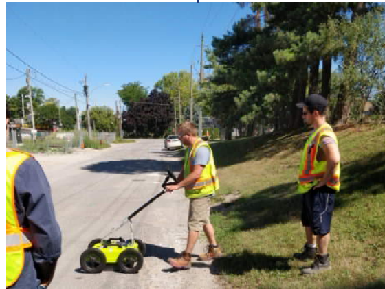
August 2022 - Completed ground penetrating radar (GPR) to identify limits of existing critical pipe to check clearances to proposed watermain
