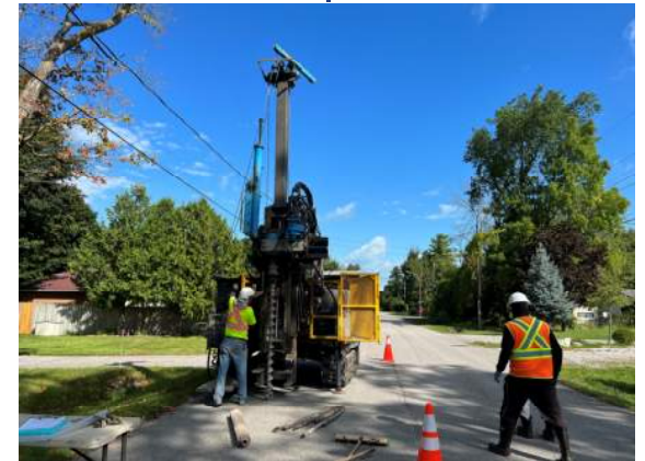
August 2022 - Completed drilling to understand the existing soils around the new watermain
