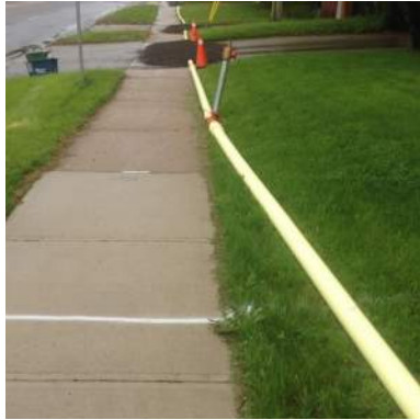
Temporary Potable Water System
