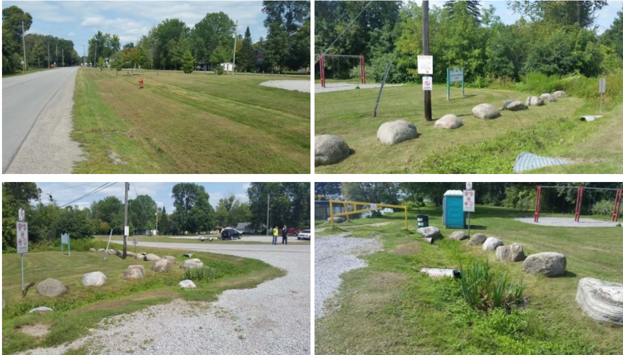
Figure 8.12: Stormwater Drainage Features around Young's Harbour Park from Upstream to Downstream: Grass swale along Lake Drive South (top left), Culverts under Lake Drive South (top right), swale between Lake Drive South and outlet (bottom left), and outlet CSPs to the Lake (bottom right).
