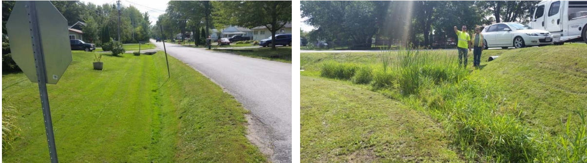
Figure 8.13: Rural Road Cross-Sections at Sunset Beach Road (left) and Waterbend Drive (right).
