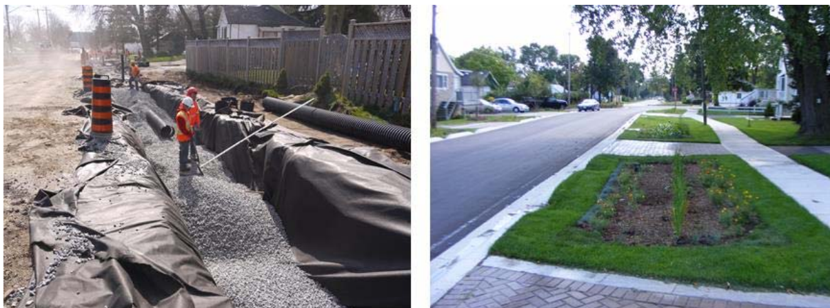
Figure 6.9: Perforated Pipe within Bioswale.
