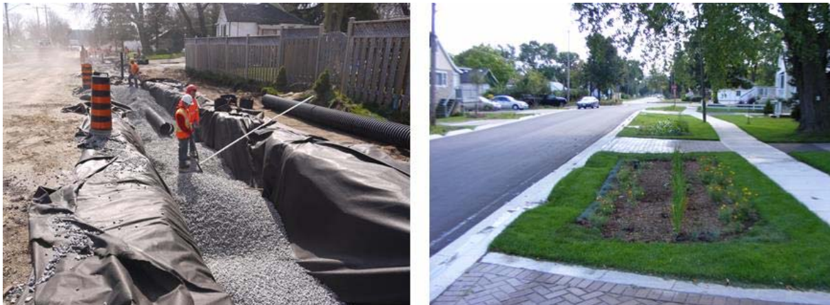
Figure 8.14: An Exfiltration Trench / Perforated Pipe System (Left: during construction, Right: after construction).
