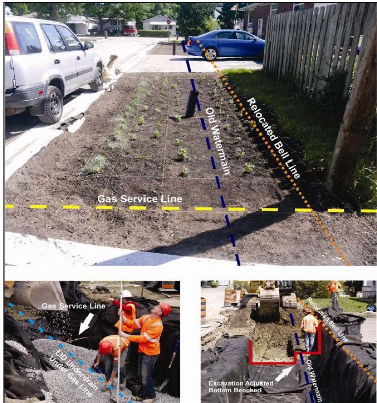
Figure 6.1: LIDs are flexible in both design and construction. Here a clear stone trench for the Lakeview Bioretention System is constructed around utilities.
