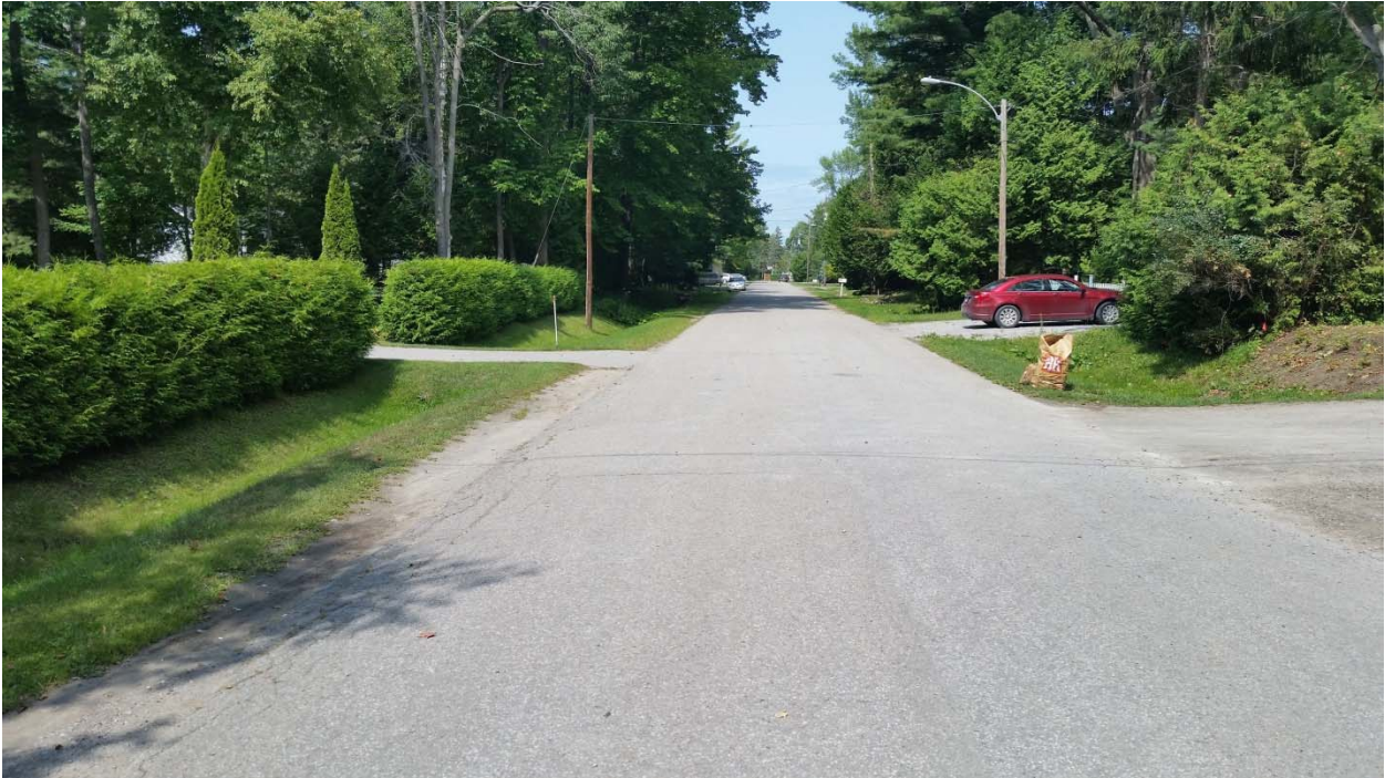
Figure 8.18: Dunkirk Avenue is a 450 m long dead-end road running south of Hedge Road approximately 200 m east of the Black River. This photo is looking north from the southern limit of the road.
