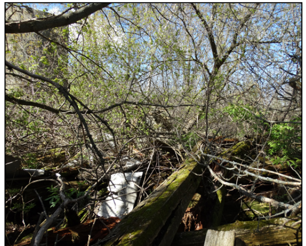
Figure 22: The barn ruins indicate frame construction with large dimension timbers and a dry stone foundation wall. The silo is a 20 th century, poured concrete type. The ruins are west of the stable and shed, at the edge of what is now a forest area.
